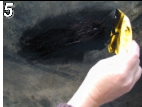
5 See "Six Easy Steps for Belt Repair" for instructions on mixing Eli-Flex. Apply to the underside of the belt. Force as much product up through the opening
